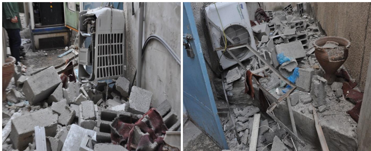
Damages at NECC three family health care centers, pre-intervention
